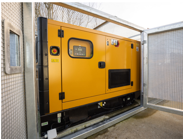
Figure 3. Diesel Backup Generator
