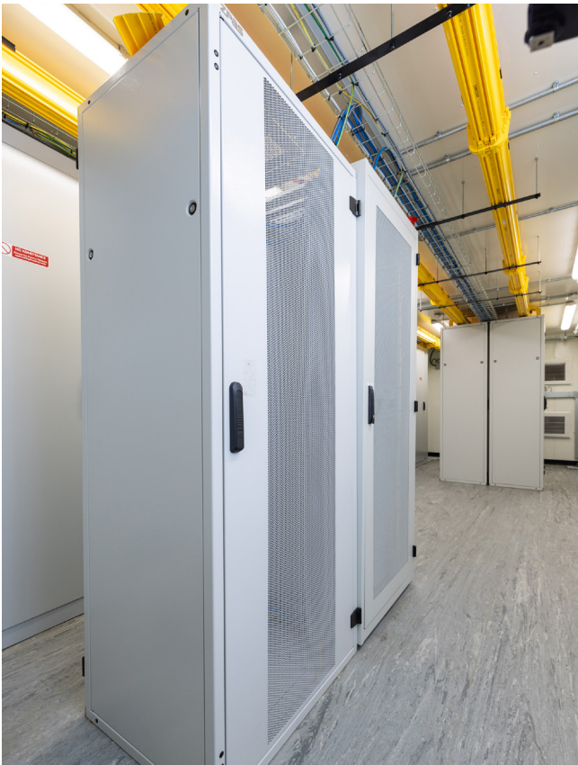
Figure 9. Typical Customer Racks
