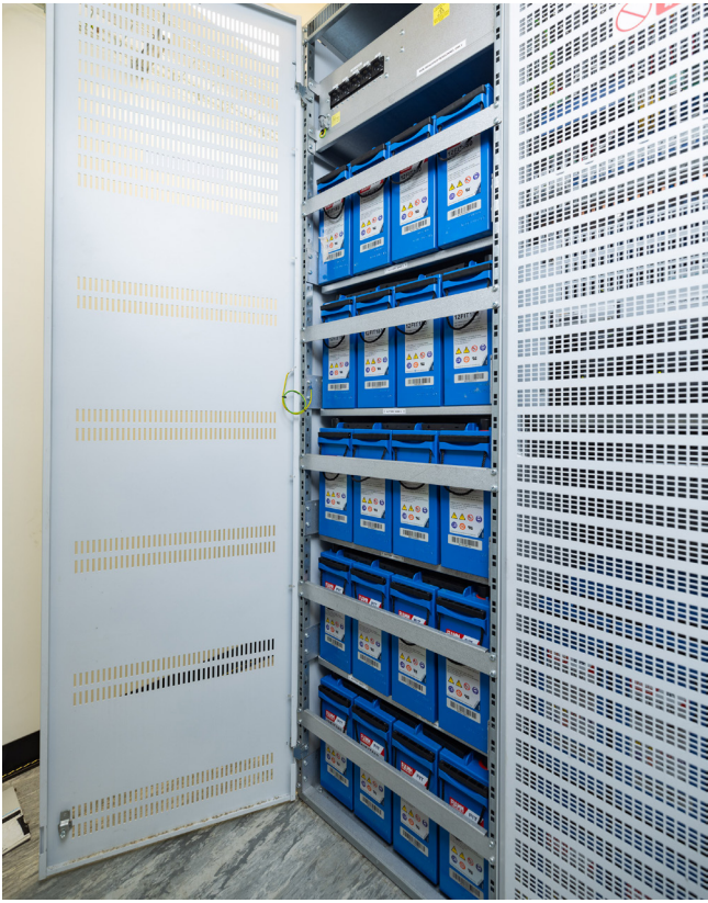
Figure 4. Typical Rectifier and Battery Cell Set up
